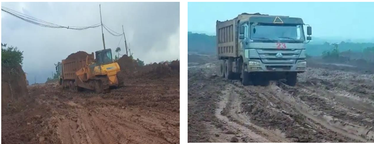
Figure 1. Project-specific field photographs of the Nhan Co bauxite mine haul road under wet-season conditions, showing surface mud formation, water accumulation, and reduced trafficability. The photographs were provided by the Nhan Co plant and are used with permission
